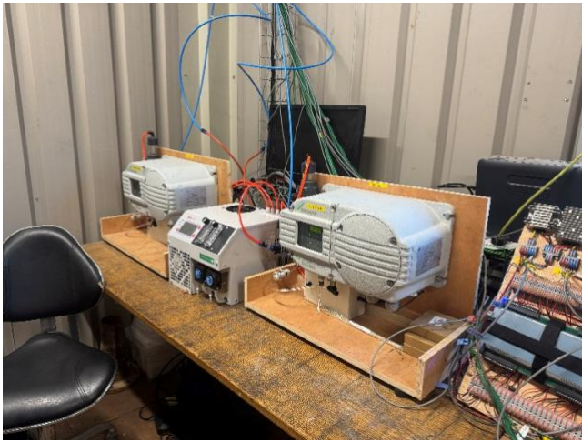
Figure 11 Gas analysis and conditioning system
