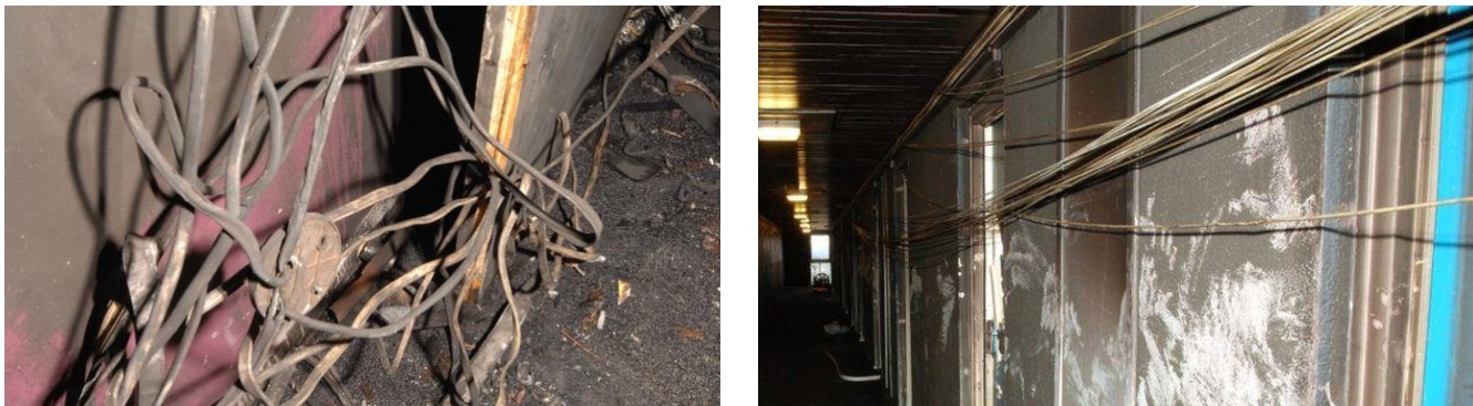
Figure 5 Fallen cable at Shirley Towers
