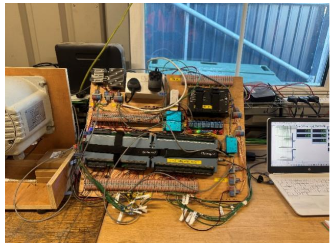
Figure 10 Data logging system
