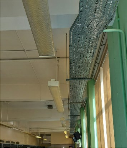
Unistruts, hangers & Cable trays
