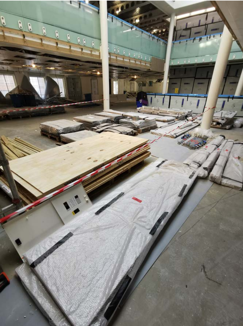
Reuse in situ material collected, sorted, protected and referenced for reconditioning and reinstallation.
