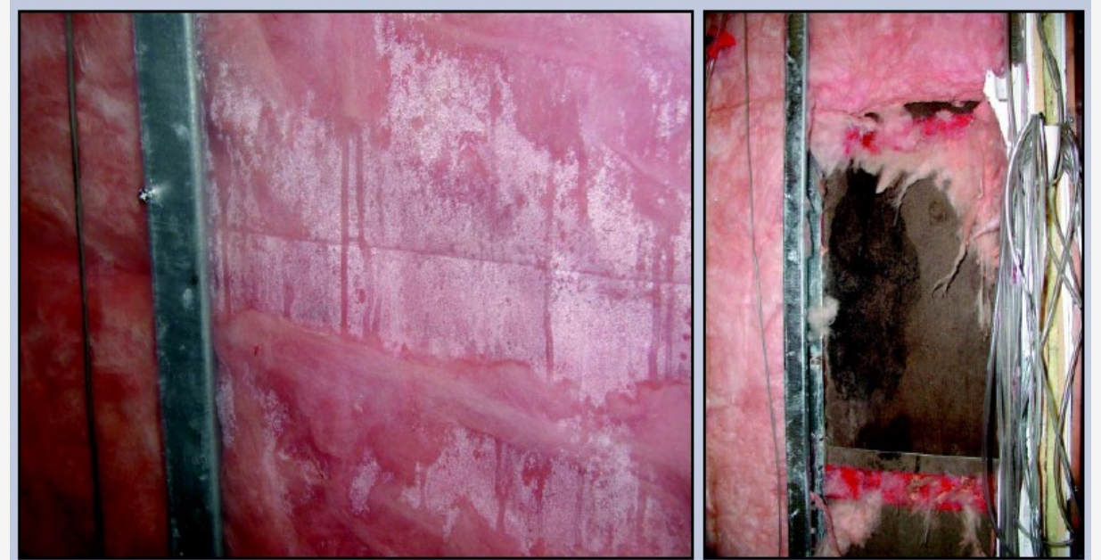
Water vapor diffusing inward during summer conditions in a cold climate (Waterloo, Canada) condensing on a low-permeance vapor barrier. The resulting damage is shown at right.
