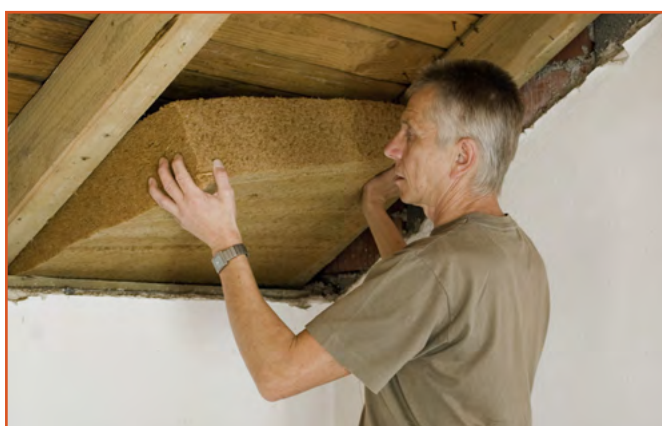
'Vapour open', breathable materials such as natural fibre insulation help to regulate humidity and improve indoor air quality
