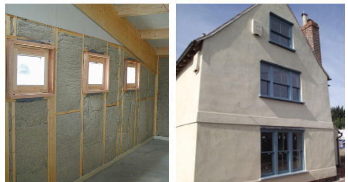
Natural fibre materials are often used in conjunction with mineral products such as lime renders.
